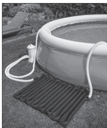
Solar Pool Water Heating
