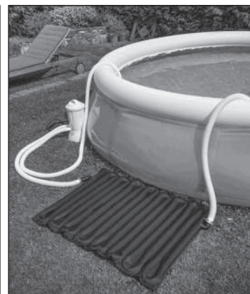
Solar Pool Water Heating
